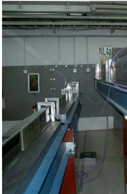
Figure 1.16: View of NGs NL4a (to the right) and NL4b (to the left) in the NG hall during the installation period. NL4a is completely enwrapped with lead ending at the position of the selector. For NL4b the glass elements have been adjusted above the bottom lead plate by means of the adjustment frames.
